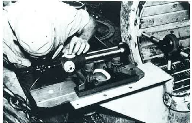
Aligning main propulsion shaft bearings on a large naval vessel with a K&E Alignment Telescope and accessory equipment. Portability eliminates the need for building accurate devices into each setup at critical points.
